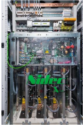
Power conversion system essential for BESS
