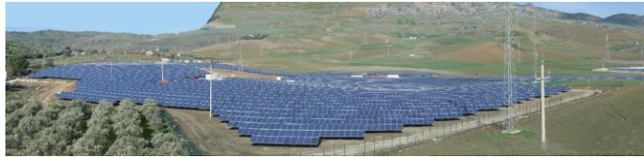
Photovoltaic power generation plant in a suburb of Ciminna, Sicily, Italy
