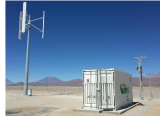
Micro-grid system in Chile
