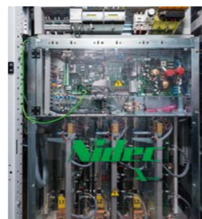
Power conversion system essential for BESS
