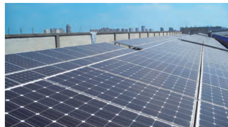
Solar panels installed on the roof Nidec (Zhejiang) Corporation's building
