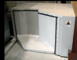
Rack door closed
