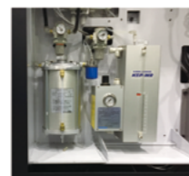
Tank for cleaning liquid is layouted in maintenance area.
